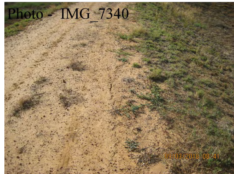
Ch. 1600 – Crack Town Side of Crest
