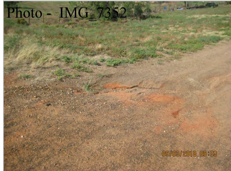
Ch 2450 – Damage Adjacent to Alama Road
