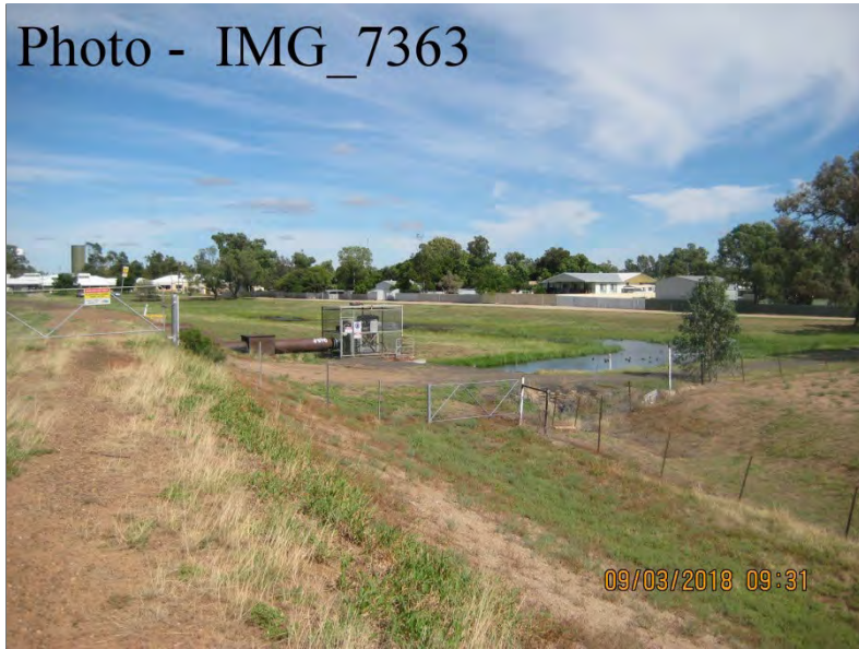
Ch. 3400 – Ponding Water at Town Side Toe
