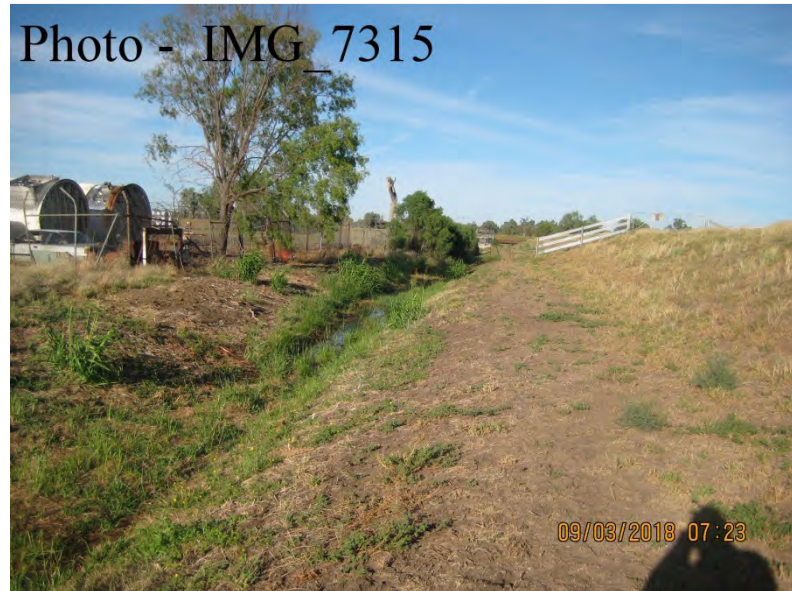
Ch. 7500 – Ponding Water on Town Side Toe
