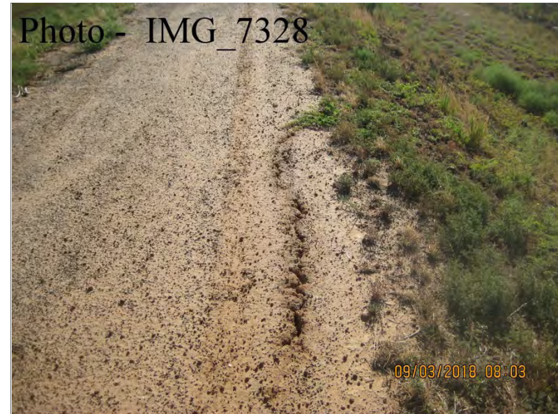
Ch 50.- Crack Town Side of Crest
