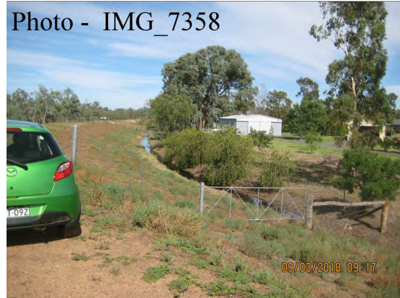
Ch 2900 – Ponding Water at Town Side Toe
